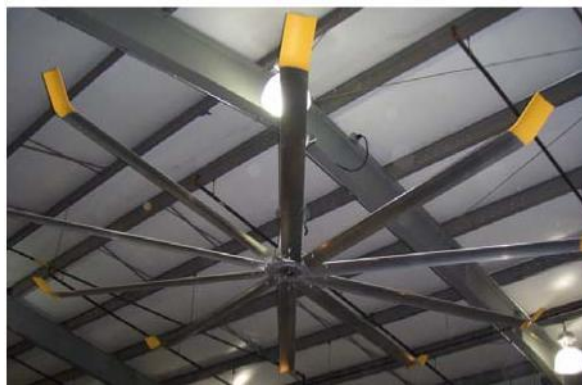
Ceiling level high volume low speed circulating air fan
