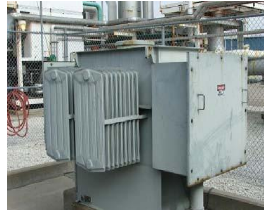
Oil filled transformer Photo source: Predictive Service
