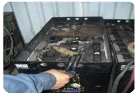
Metal chain near battery terminals Photo Source: Predictive Service
